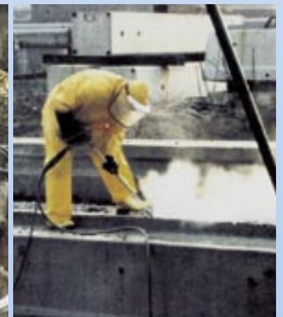
Exposing of reinforcement bars
